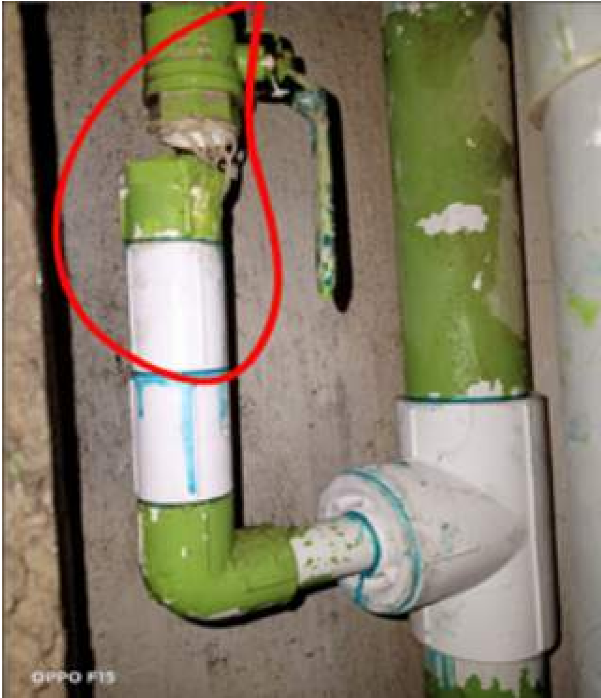
Branch pipe failure. Pipe sheared at this location.
